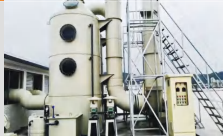
⦿ Application scenario of waste gas purification
